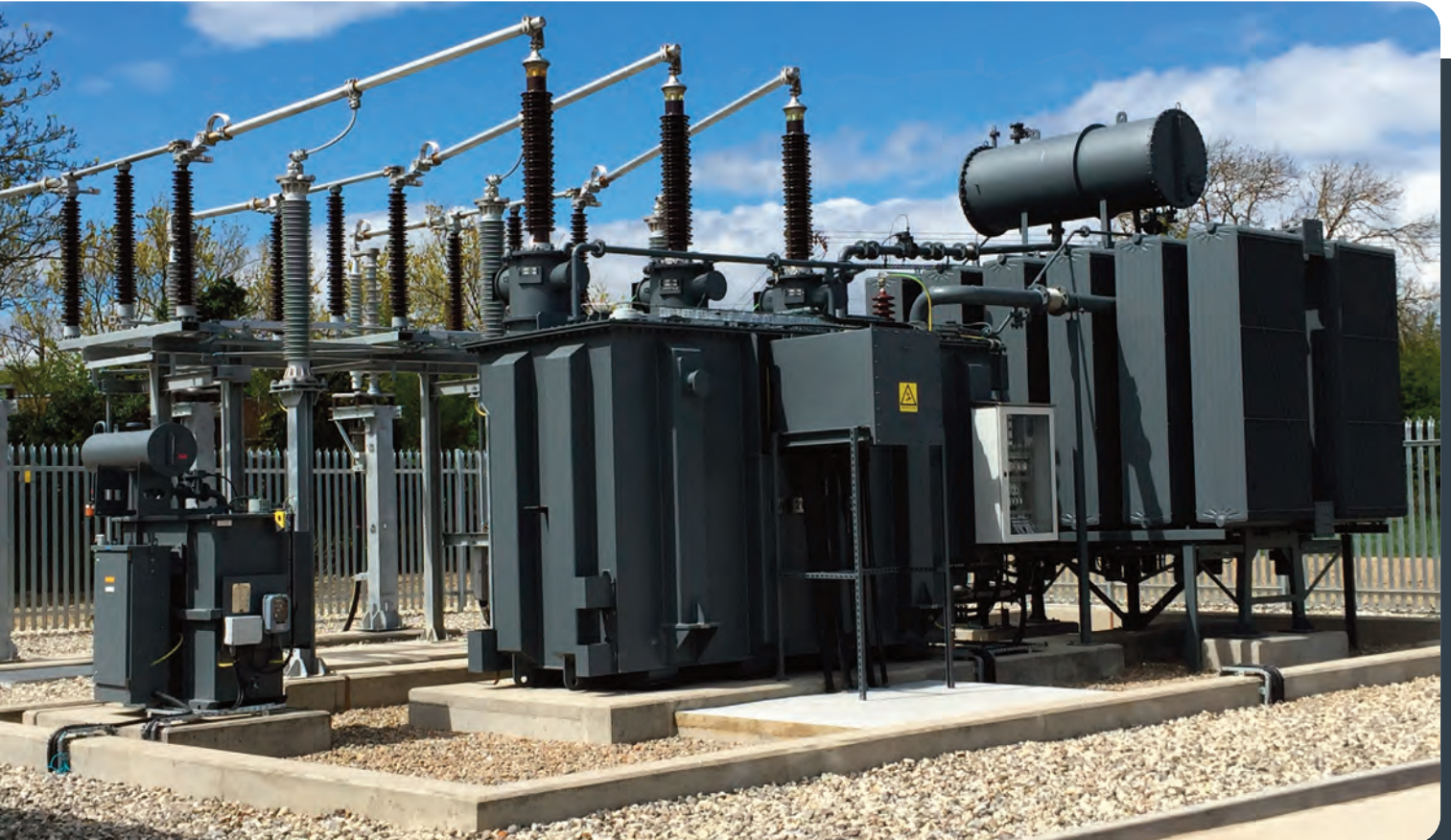
50MVA Wilson Power Transformer at Melbourne Grid
