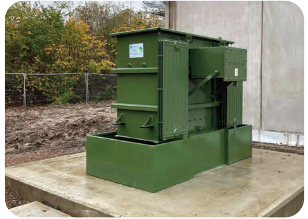
1MVA Auxiliary Transformer at Erskine
