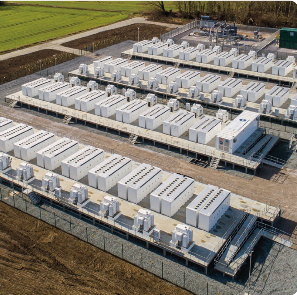
Pillswood, Cottingham 98MW/196MWh
